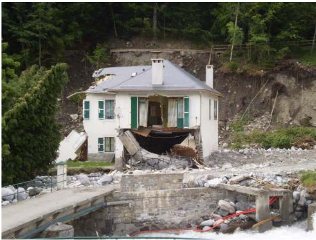
Fig. 1. House destroyed by the Bastan flood on the 18th of June 2013 in Barèges, in the Hautes-Pyrénées (photo taken on the 03/07/2013, S. Carladous).
